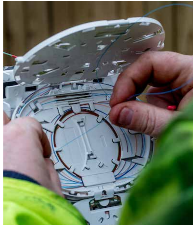
Engineer Graham Wray carries out fibre splicing and testing, simply put, fibre optic splicing involves joining two fibre optic cables together.
